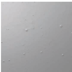
Surface defects due to outgassing
